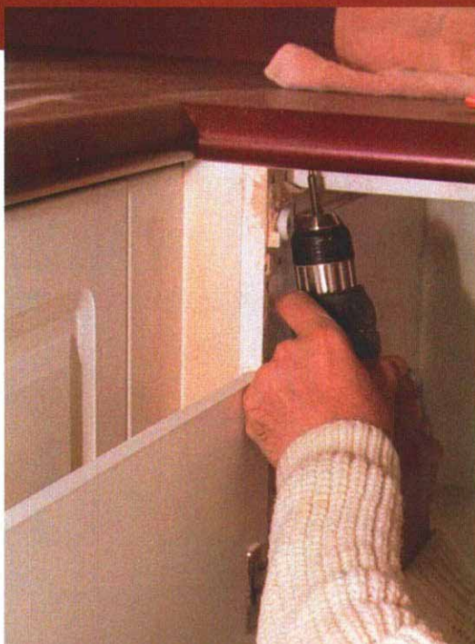
Don't pierce the top after all that work. Use 1/4-in. #8 wood screws to fasten the countertop to the cabinets and to the 2-in. wide strips applied along the tops of the cabinets.
