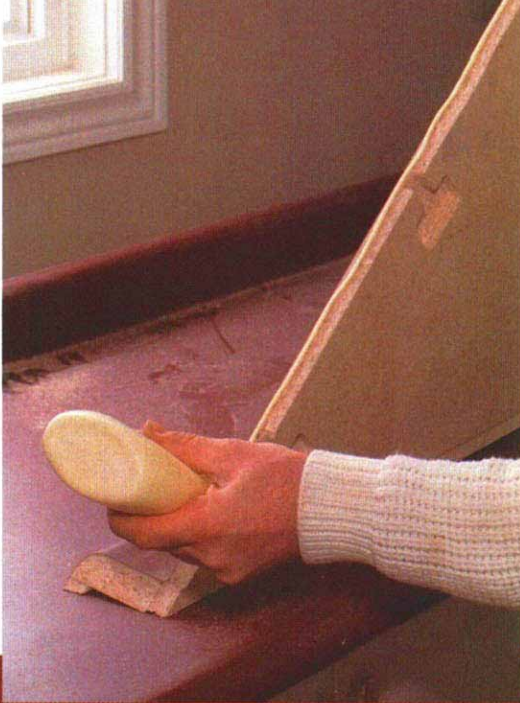
Join miters with waterproof glue. Too much glue in a joint will swell the particleboard, leaving a bump in the surface of the countertop. Use just enough to produce a small amount of squeeze-out on top.
